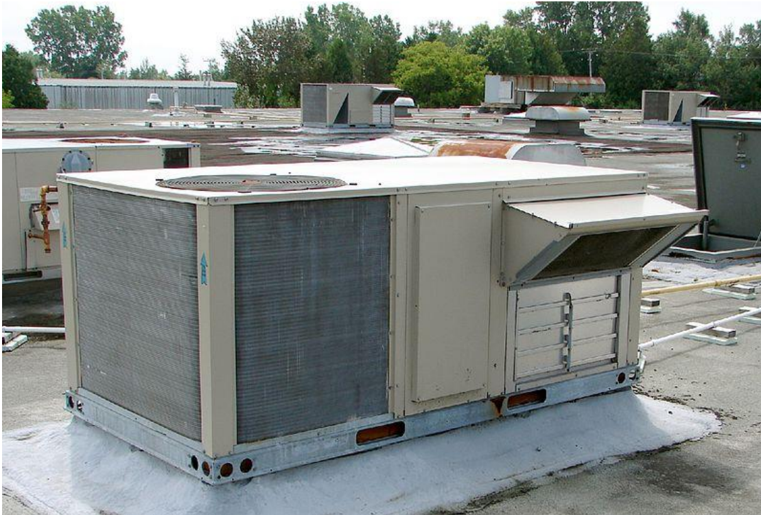
Rooftop Units (RTUs)
