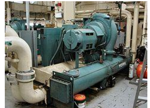
Chillers and boilers
