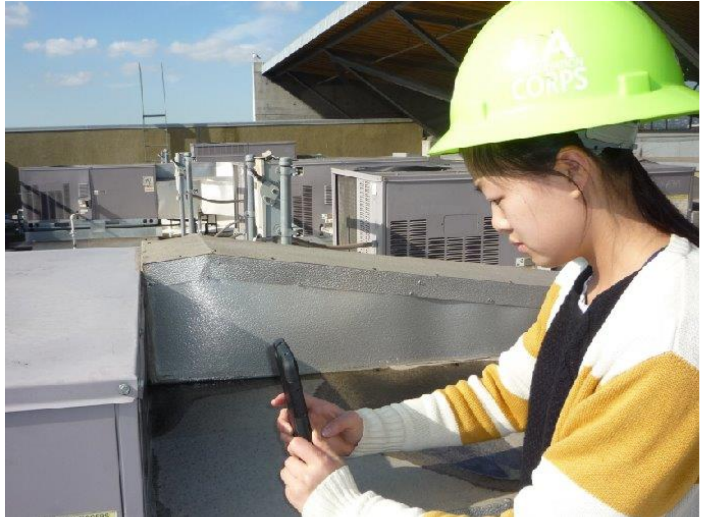
Student Performing Energy Audit, Los Angeles USD, CA Credit: Los Angeles USD
