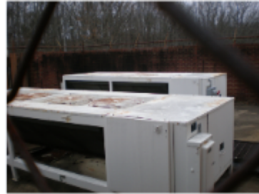
ECM 4c-1 – Dillard Elementary School HVAC Upgrades
