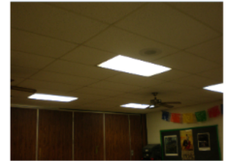
ECM 1A – Lighting Retrofits
